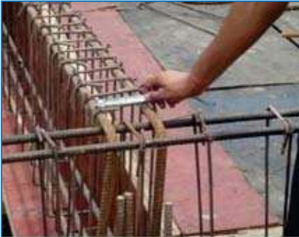
Inadequate hook length and absence of 135° angle reported in CBRI Report No. 2
