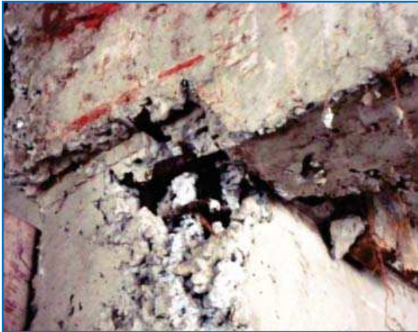
Exposure of Reinforcement Column cap (Report No. 9 - Tower 20, 4 th floor)
