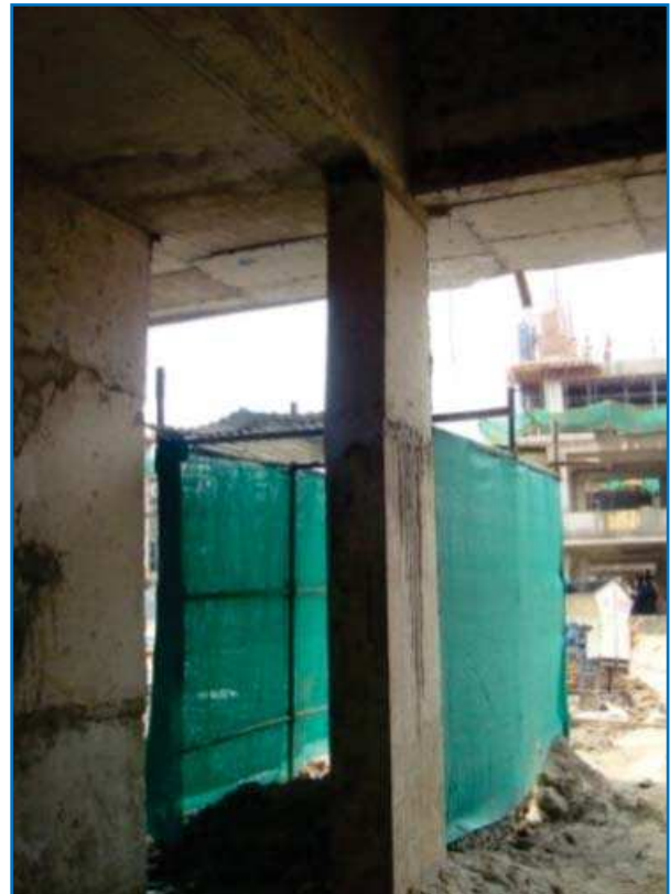
Bent up Column in the Basement of Tower-3 (Report No. 3)
