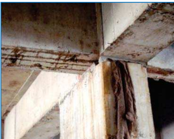
All in one (Exposed Steel, Hole in Beam Column Junction, Insertion of Jute Bag) Tower 15 as reported in CBRI Report No. 9
