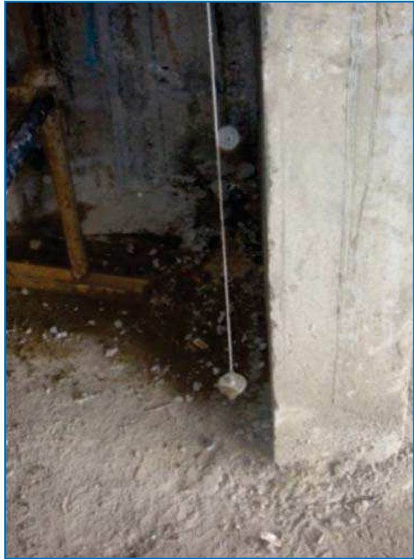
Column Out of Plumb in the Basement of Tower-3 (Report No. 3)
