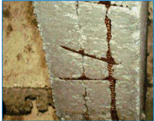
Reinforcement is seen in beam bottom (Report No. 9-Tower 23 - 6 th Floor)
