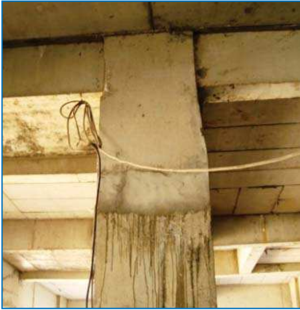
Tower -10: Tapered column (LB) Report No. 9
