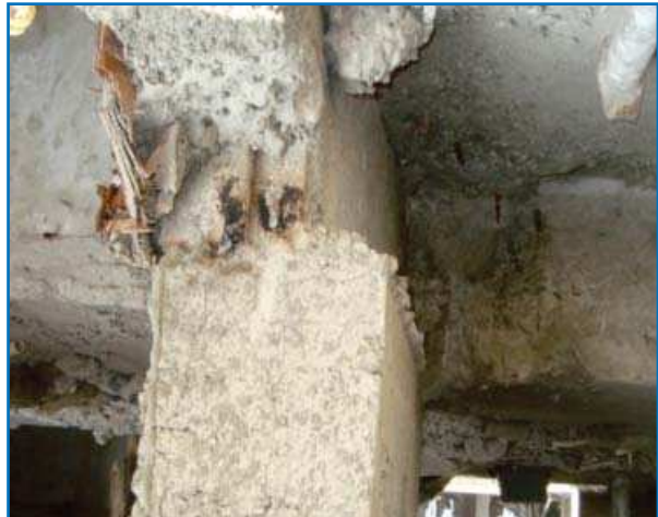
Exposed bars in the joint (- Report No. 9-Tower-6)
