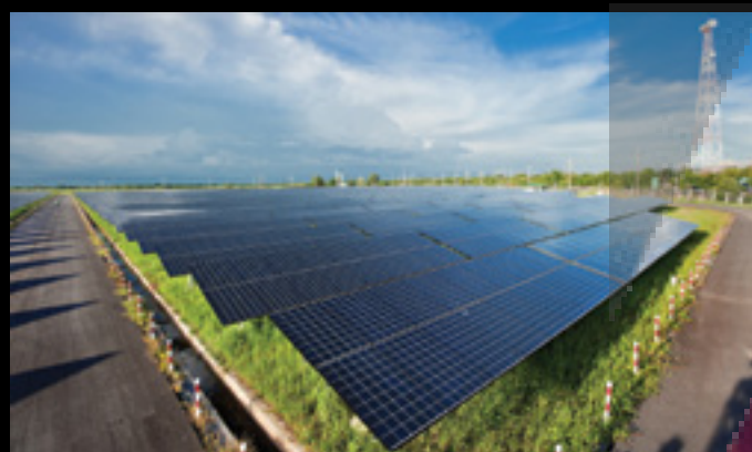
Solar panels for energy saving
