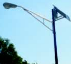
Power saving street light
