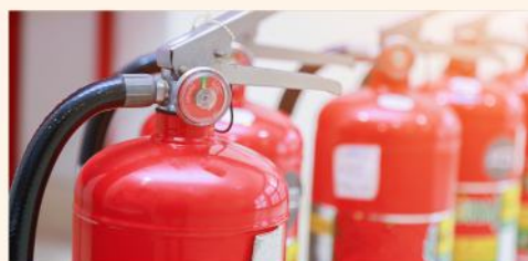
Firefighting & alarm system
