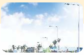
LED STREET LIGHTS
