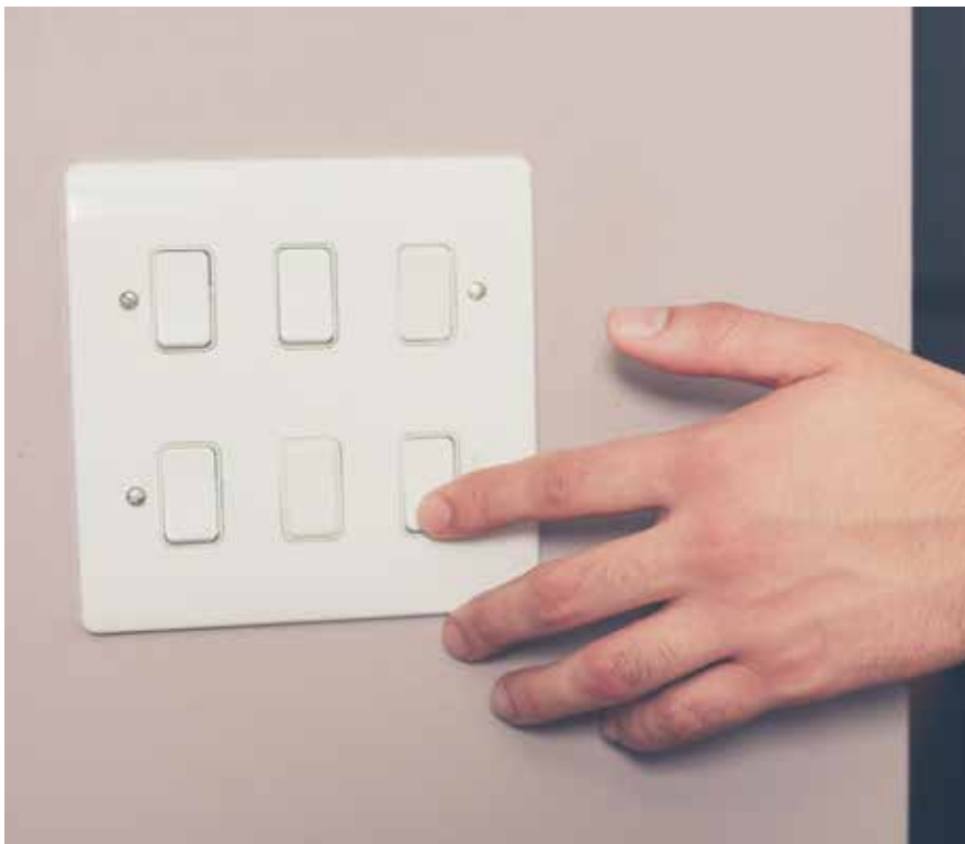
Modular switches and concealed copper wiring
