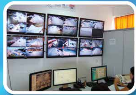
Surveillance System in Common areas & Parking
