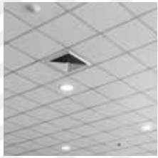
CEILING GRID FALSE CEILING
